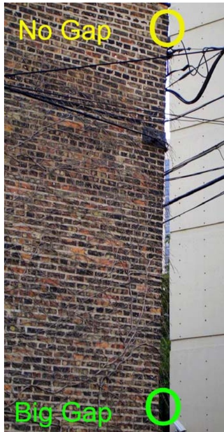
The leaning Carriage House
